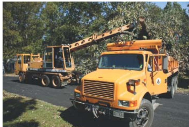
Just after Isabel hit, residents woke to a multitude of crews from Henrico's Public Works and Utilities departments removing debris throughout the county.
